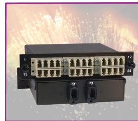
Model 6012 Two 12-Fiber MTP/MPO inputs break-out to 24 LC outputs (24 Simplex or 12 Duplex)
